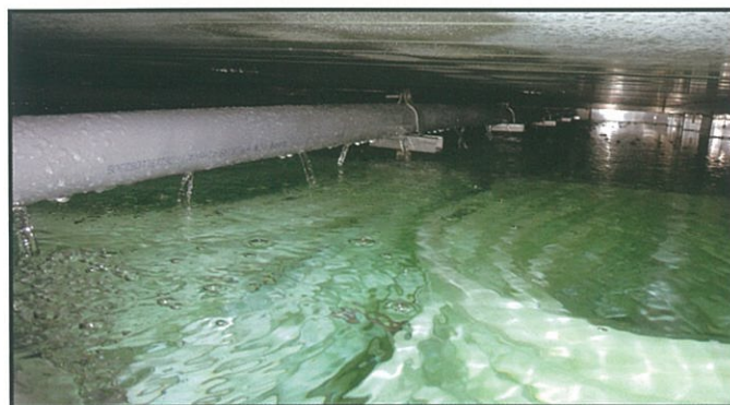
儲冰槽內融冰 Ice Melting in the Ice Storage tank
