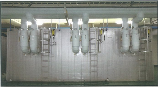
室內儲冰槽 Indoor Ice Storage Tank
