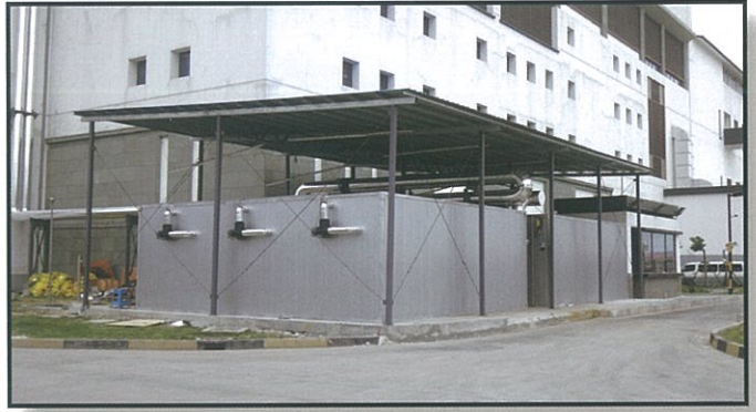
戶外儲冰槽 Outdoor Ice Storage Tank
